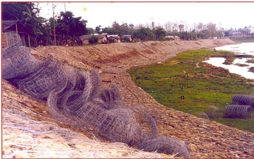
Anti-erosion works under execution to protect Kushiabil and Durgajan villages at Dimapur on River Dhansiri(South) in Nagaland
